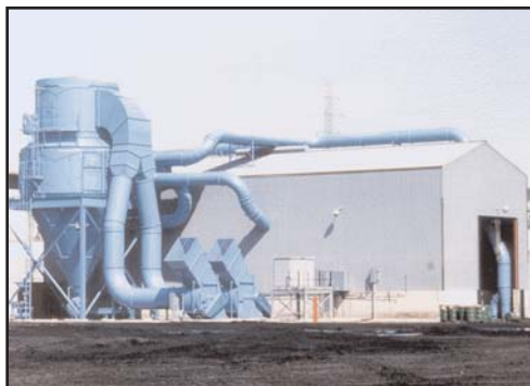
This 984RF12 is collecting coal dust from bottom dump railroad cars.
