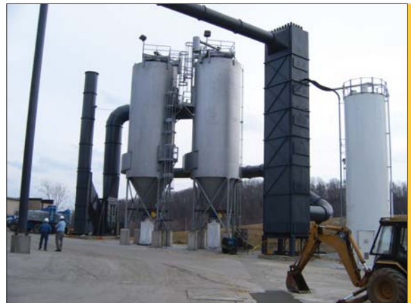
484RF two high temperature collectors on secondary aluminum processing
